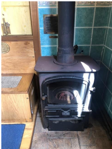
▲ Stove starboard side
