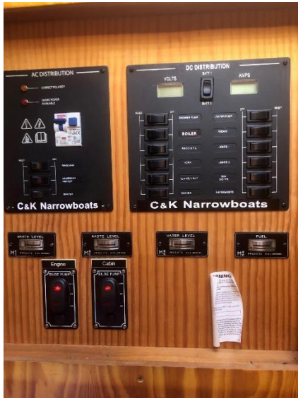
▲ Switches and gauges
